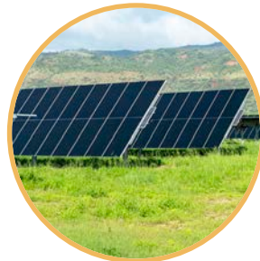
Solar panels at PMRF.
